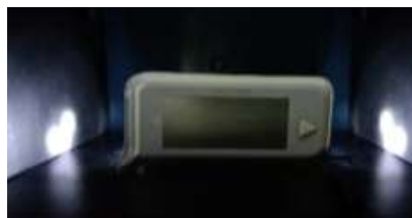
(Emergency LED when power failure)
