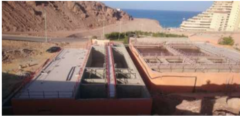
Fig. 2. Extended W.W.T.P at red sea resort & its expansion (executed by researcher).
